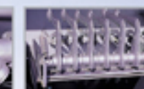
Emergency control valve can be controlled from above and flow stopped in case of emergency
