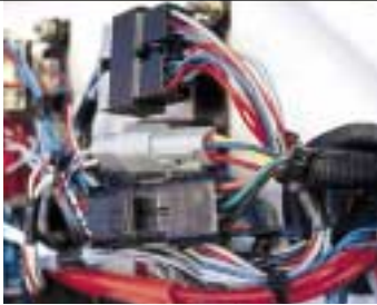
To speed troubleshooting, wiring is color coded and numbered.
